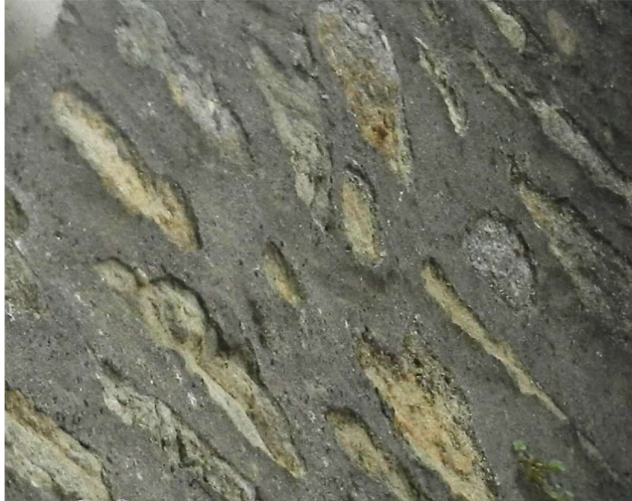
Photo 16 – stone erosion north elevation
