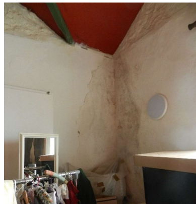
photo 27 – damp SE corner R203
