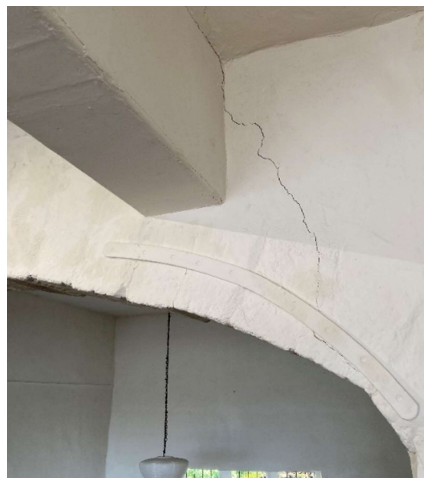
Photo 23 – Cracked arch gallery side
