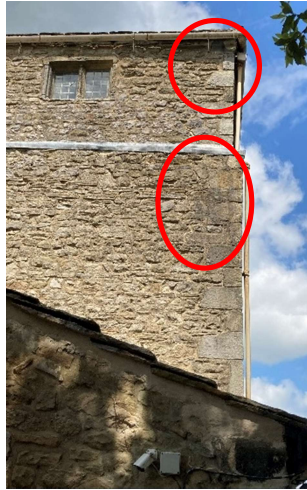
photo 17 – Location of open joints & crack in mortar in south elevation of tower
