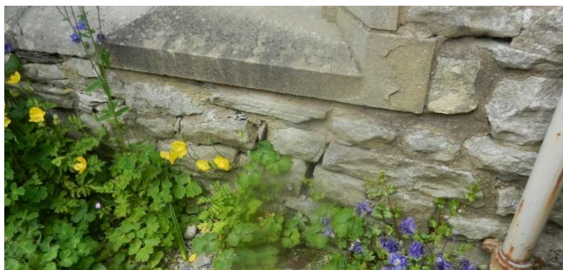
photo 21 – open joints under WG10
