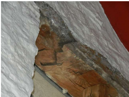
photo 26 – split imber lintel R203
