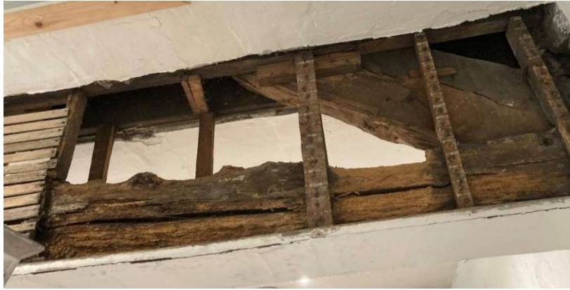
Photo 25 – Truss beam is in poor condition with a large shake and friable timber
