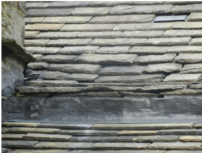
photo 5 – dip in roof over east wall in R201
