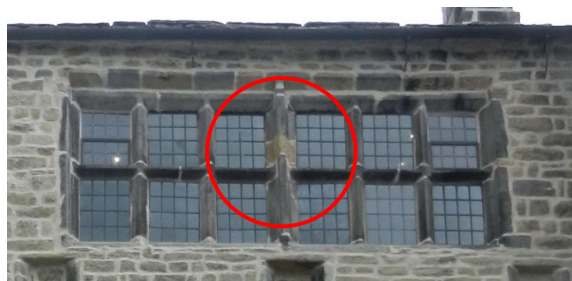
photo 15 – stone erosion to mullion
