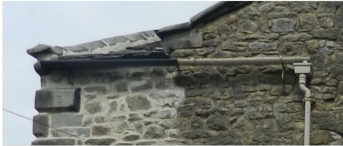
photo 13 – gutter to south elevation to be monitored for overflowing
