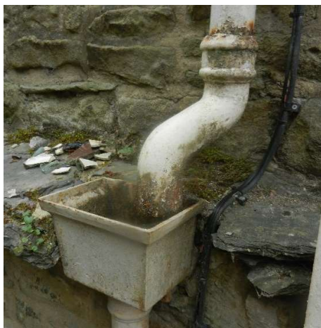
photo 11 – corroded rwp & hopper west elevation
