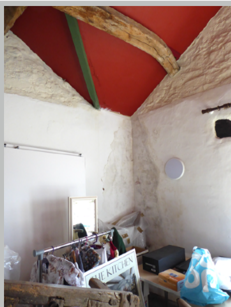
Plate 12. Damaged internal plaster
