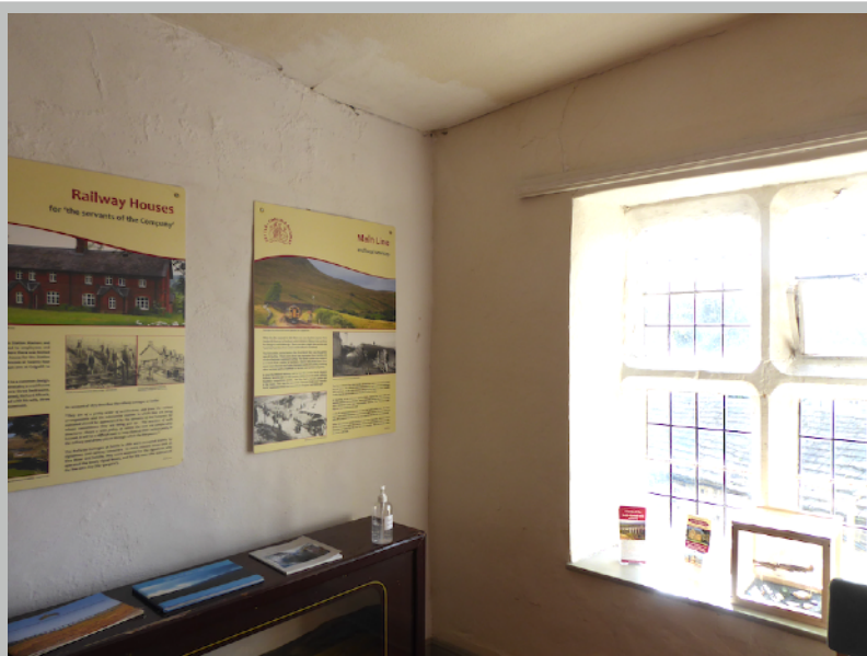
Plate 11. Damaged internal plaster
