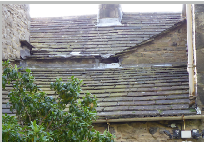
Plate 10. Area of roof to be repaired
