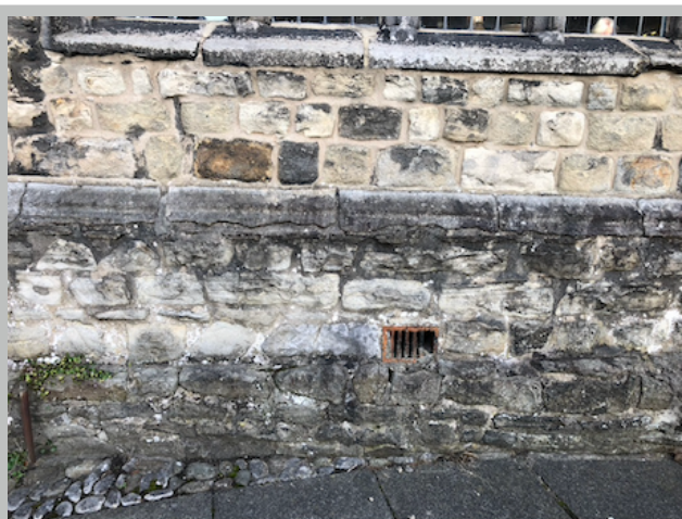
Plate 3. Sample pointing and damaged vent grill
