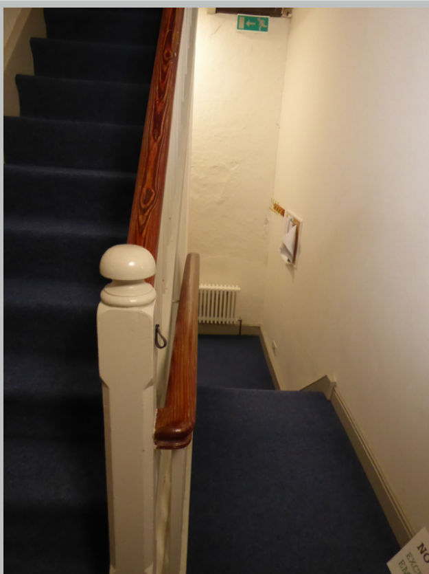
Plate 19. Staircase to be replaced
