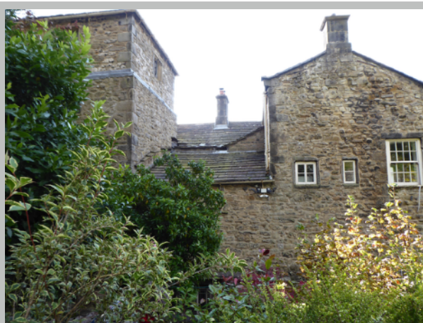
Plate 9. Area of roof to be repaired
